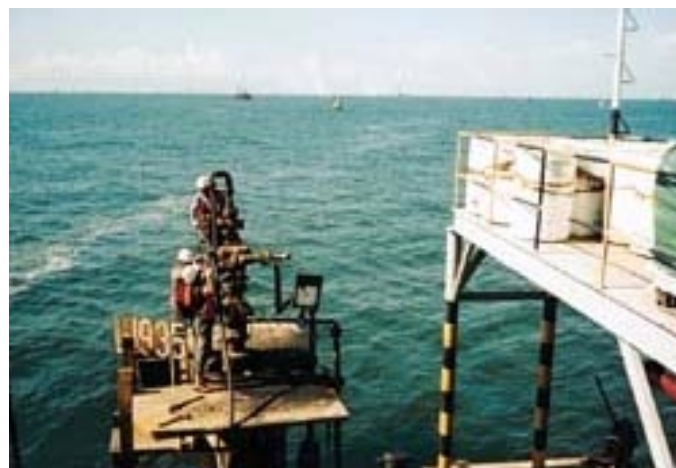
A triplex pump on a self-propelled barge was used to inject the microbial treatments (Fig. 2).
