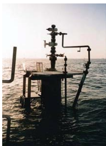
Small well head platforms are common in Lake Maracaibo (Fig. 1).
