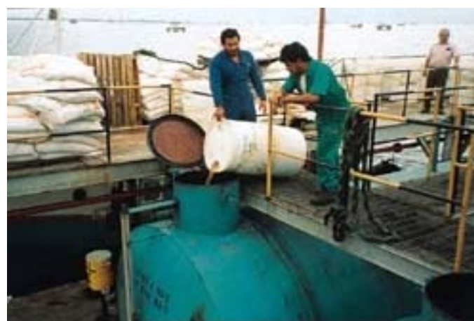
Workers pour a microbial scale and corrosion inhibitor into a mixing tank (Fig. 3).
